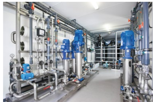
Process water treatment
